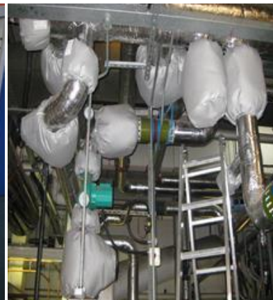
Hot water Pipe Lagging
