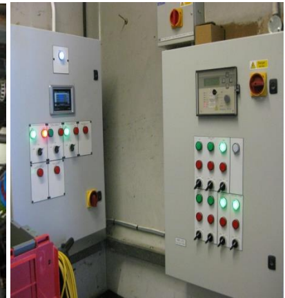
Heating control system
